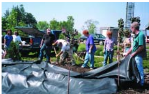
Members of the Eastern Iowa Pond Society pitched in to set the pond's liner.
