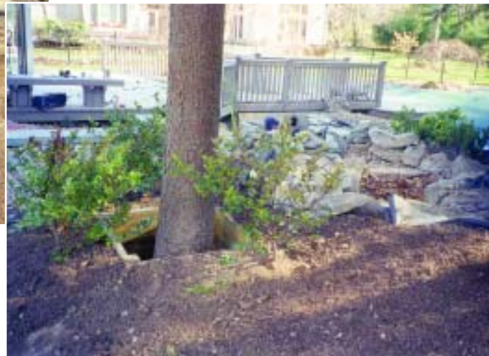
Backfill soil against the boxed tree well and landscape to hide the well.
