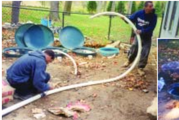
Plumbing, which will bring water from the pond's bottom drains, is coupled together with fence coupling. The plumbing is then buried to exit water into the filtration system (the vats in the background). Care is taken to prevent elbows in the plumbing line that might trap air and inhibit the function. Also, the plumbing will be buried at no higher an elevation than the pond's water level. (Use a surveyor's level, if necessary, to determine this.)
